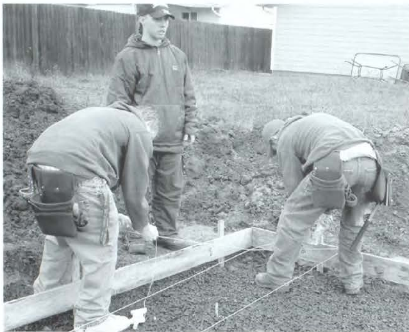
Mark the spots, junior Erik Wooton and senior Kevin Dugan prepare for the foundation pour as junior Jesse Shanklin III looks on. The construction class worked hard to build a house for Habitat for Humanity.
