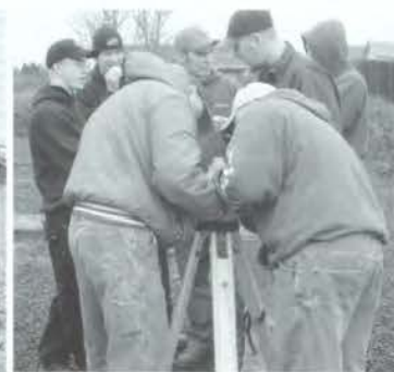
Puttin' it together, Mr. Frazier and junior Cody Miller assemble the transit as other class members observe. The transit is used to make sure the job site is level.
