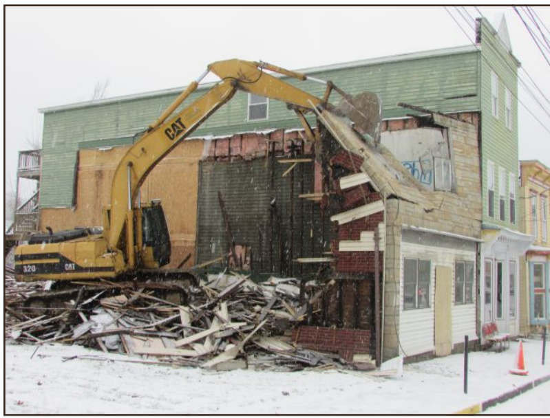
Kingwood Council worked more than a year to have this Price Street building's condition addressed.
