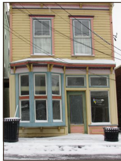
Kingwood is trying to have the Sweet Annie's building on Price Street addressed. The first floor has collapsed into the basement.
