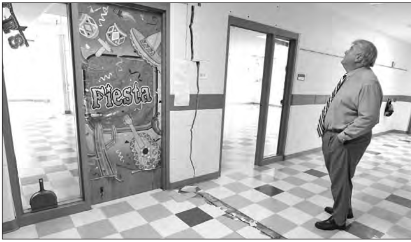
Gillespie School District superintendent Paul Skeans shows off cracks on the wall and floor inside the Benld Elementary School caused by mine subsidence, leading to the condemning of the building in Benld, Ill.
