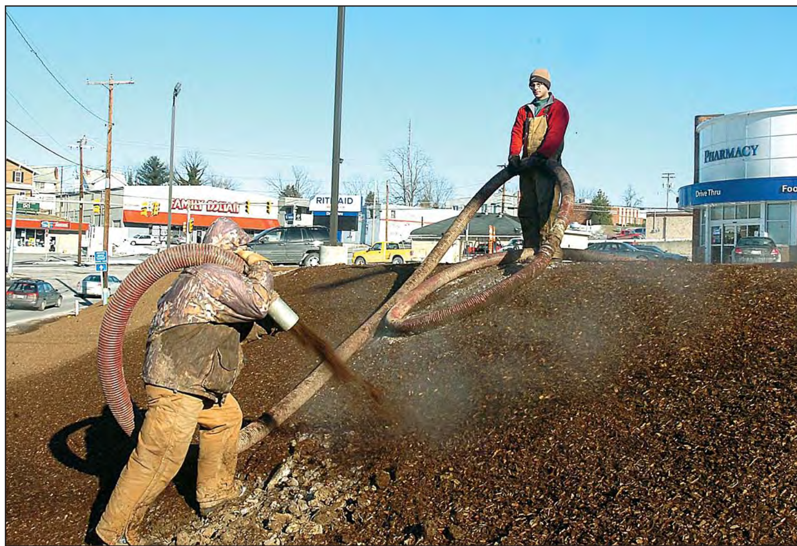
Weaver Express Blowers , of Sugar Creek, Ohio, blow mulch at the new Rite-Aid store in Westover across from Westover Exxon on Friday. Keith Weaver
