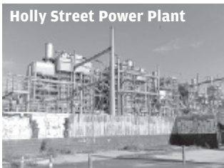
Holly Street Power Plant
