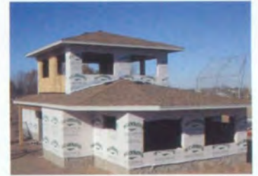
The new FLAAA building at Fenway Fields is under construction this year. "I thought it was a good experience to build a real building," commented Michael Pleski (12). Building it was a lot of work.
