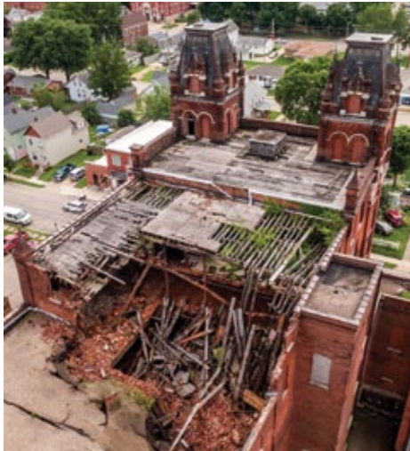
The roof collapsed on the historic Dubuque Brewing and Malting building in downtown Dubuque following heavy rains. Photo by Dubuque Aerial Media.
