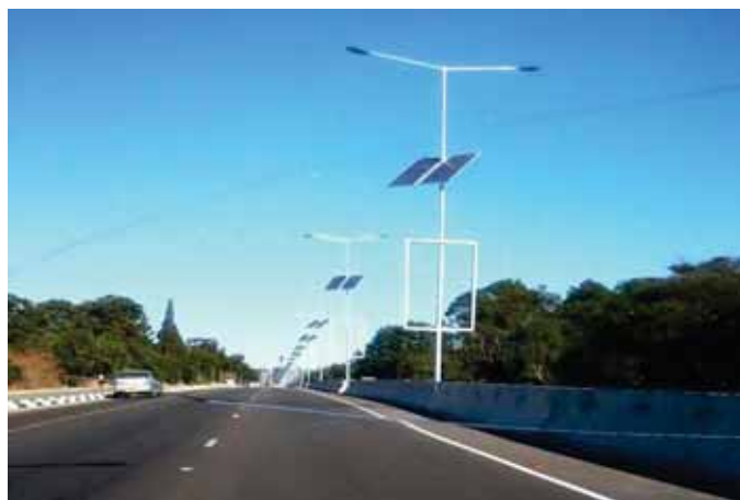
Figure 4. Street solar lighting project in Harare
