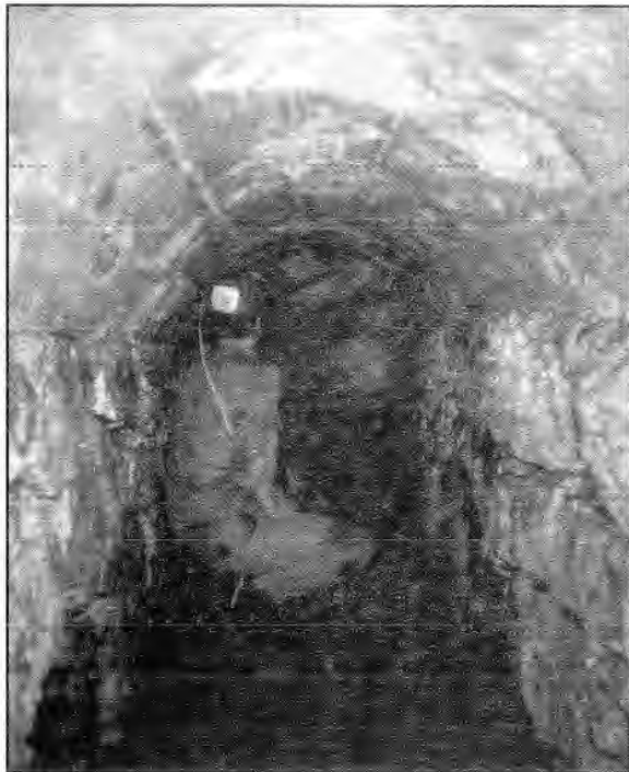
Fig. 2 Interception tunnel in the Citàgol aqueduct (Mezzolombardo - Trento). Pictures by the author.
