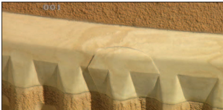
A close-up of the foam crack that has delayed liftoff for more than a month.
