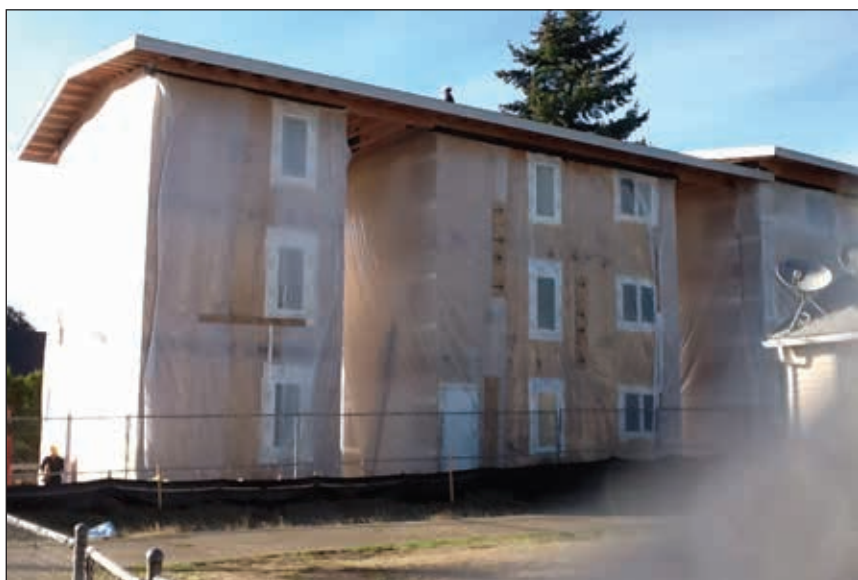
The pre-fab, modular design of the Kah San Chako Haws apartments in Southeast Portland's Lents neighborhood required only three days of on-site construction, yet the building earned LEED Gold status for sustainability. COURTESY OF NAYA FAMILY CENTER
